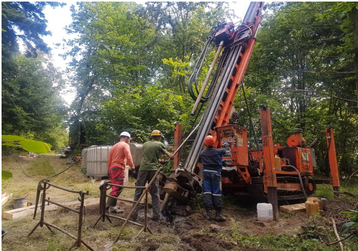
Drilling the Jasenie prospect where a new gold tungsten resource was announced during the year.
